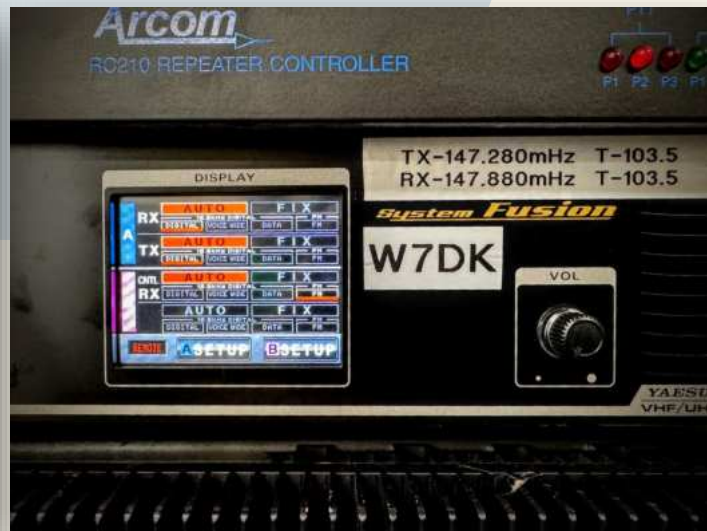
Closer view of the DR-2X programming screen This new machine replaces the decades-old GE repeater that was in the rack for many years.
